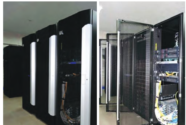
HPC Infrastructure at NBAII, Bangalore
