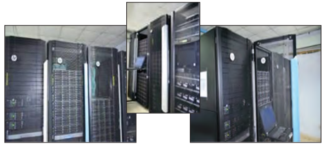
HPC Infrastructure at NBFGR, Lucknow
