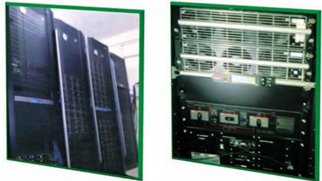
HPC Infrastructure at NBPGR, New Delhi
